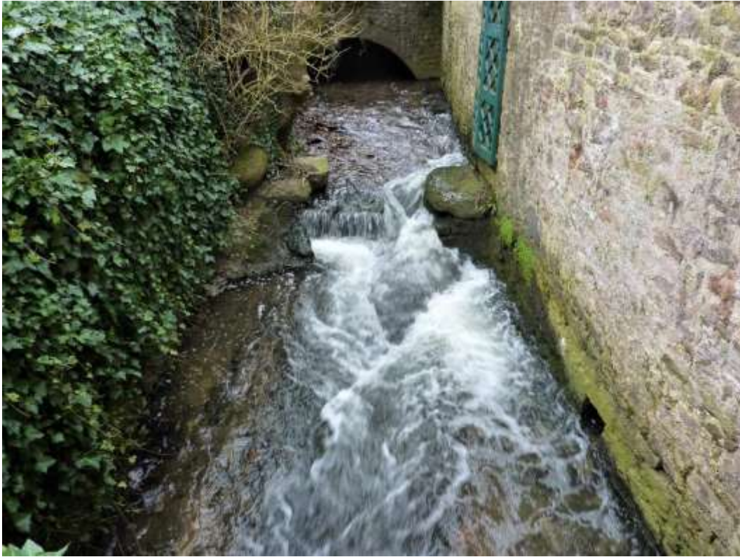
Figure 10: Small but potentially significant: a weir in the torrential bypass channel at Middle Mill
