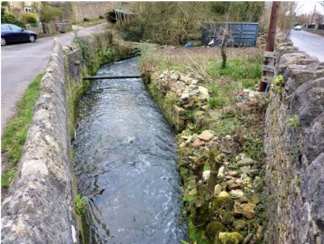
Figure 7: Looking downstream from Back Lane bridge, with deteriorating retaining walls on the RB
