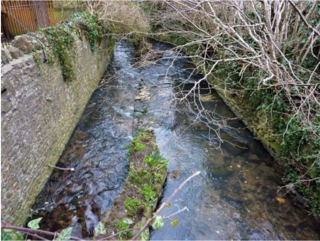
Figure 8: A mid-channel wall which is probably damaging the river's ecology in low flows
