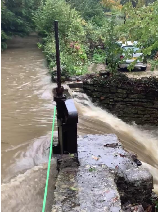
Figure 20 - River Sheppey spilling from the weir at Weirside
