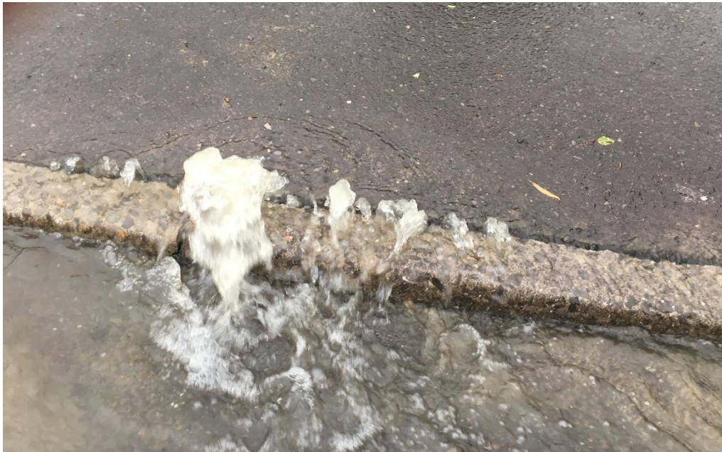
Figure 17 - Cracks in Long Street from which water was reported to be emanating.
